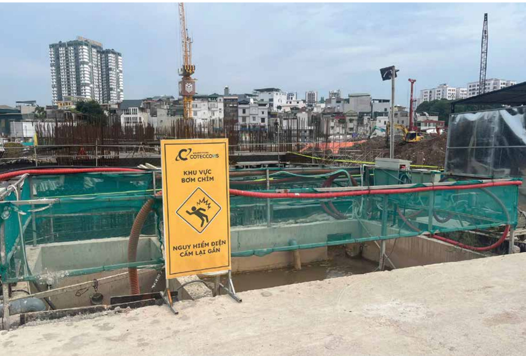
Wastewater treatment system at the Cao Xa La project in Hanoi.
